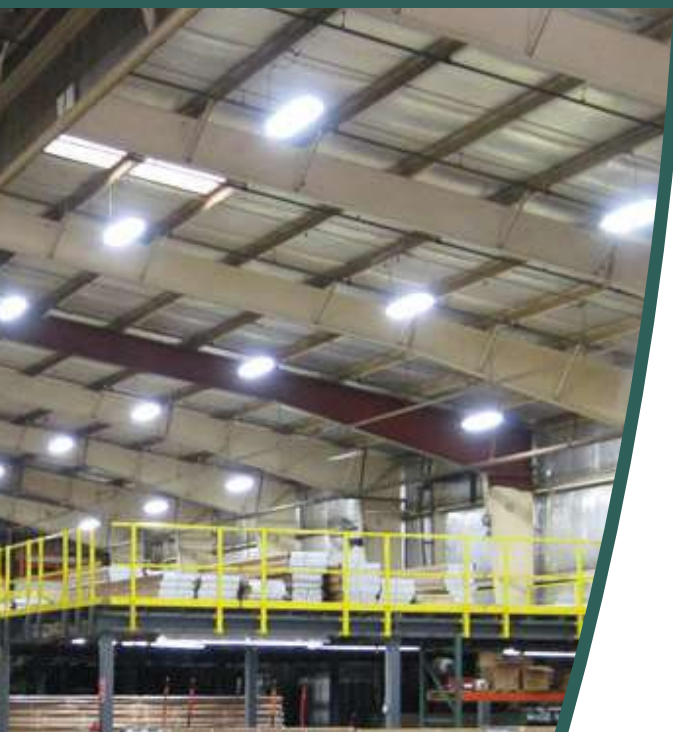
NEW WAREHOUSE LIGHTING
