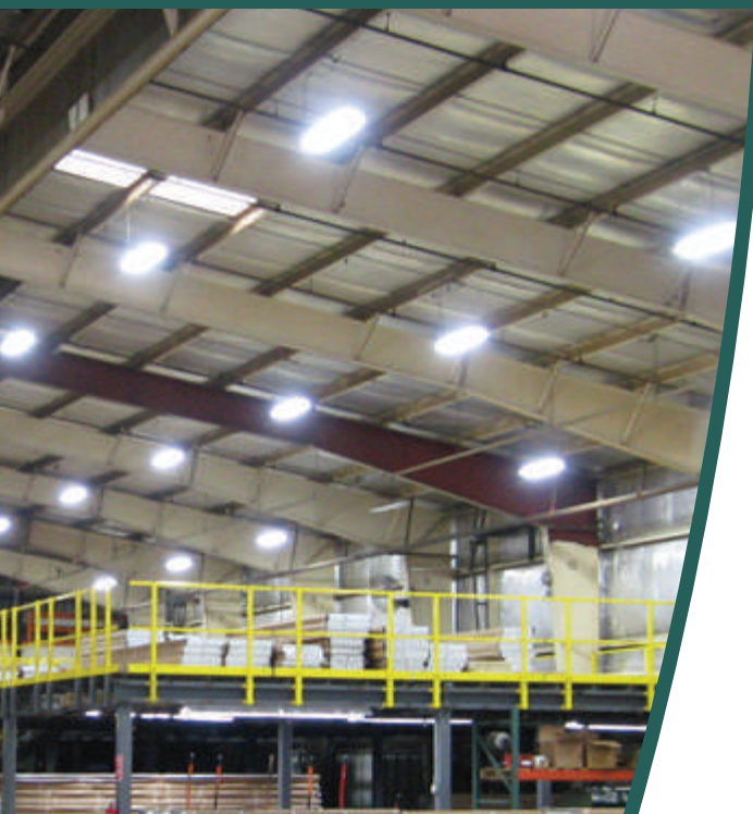
NEW WAREHOUSE LIGHTING
